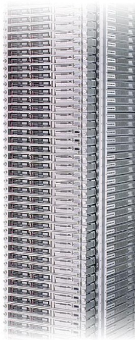
Figure 1: Deployment of ultra-dense 1U ProLiant DL360 servers in a telco rack
