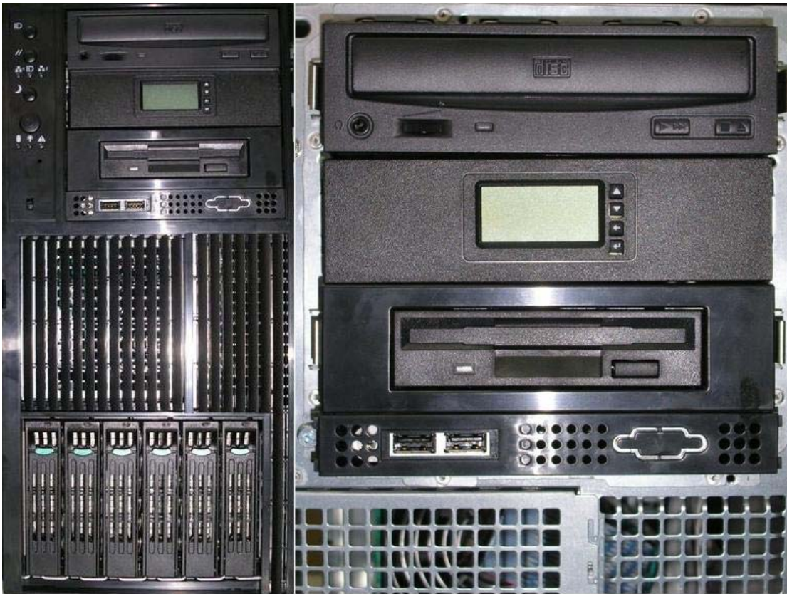
Figure 10. SKU3: Pedestal Server Installation
